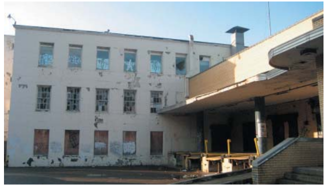
With nearly 80-thousand in county brownfield cleanup funds and nearly a half a million in Restore NY funds, this eyesore in Johnson City will hopefully be demolished soon.
